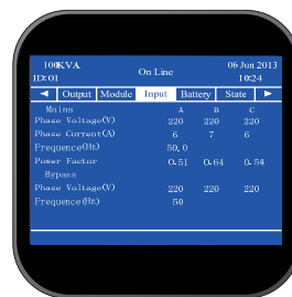
UPS Cabinet Control Panel
